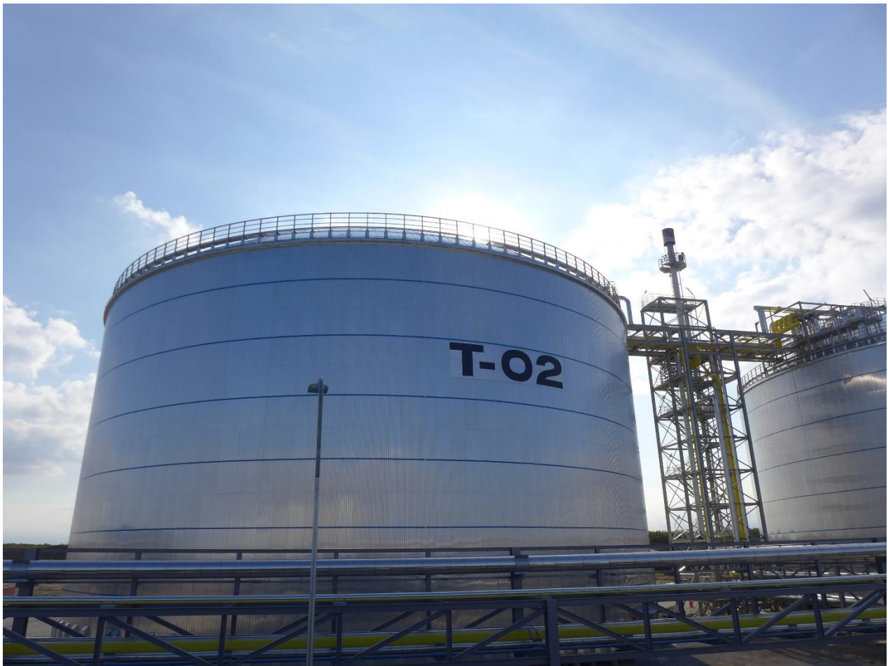
Figure 20. Refrigerated liquid ammonia storage tanks. Source: Proton Ventures.
